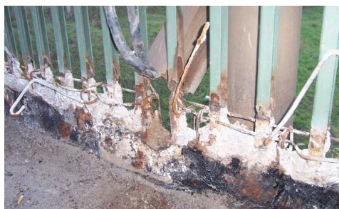
Photo 10 - Damage in the pedestrian fence
