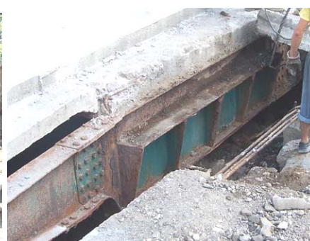
Photo 6 - The steel structure corrosion
