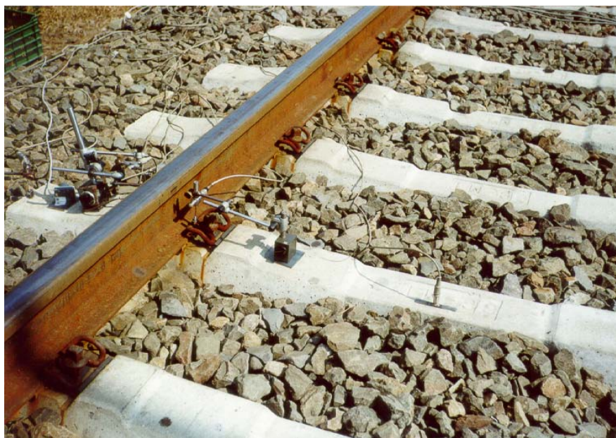
Figure 2: Superstructure of the left track and the inserted sensors for displacement and vibration
