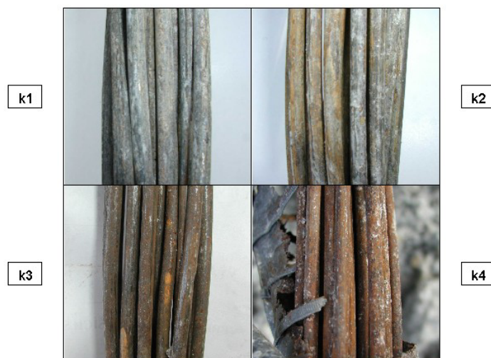
Fig. 8: Four groups of corrosion
